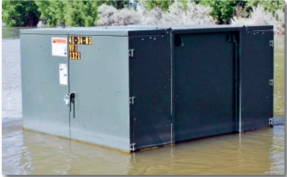
Capital Electric has many flooded facilities including this vacuum fault interrupter, which sectionalizes lines so that only a few people are out of power in case of an underground fault. Crews will be inspecting, cleaning and replacing facilities as needed when the floodwater recedes.
