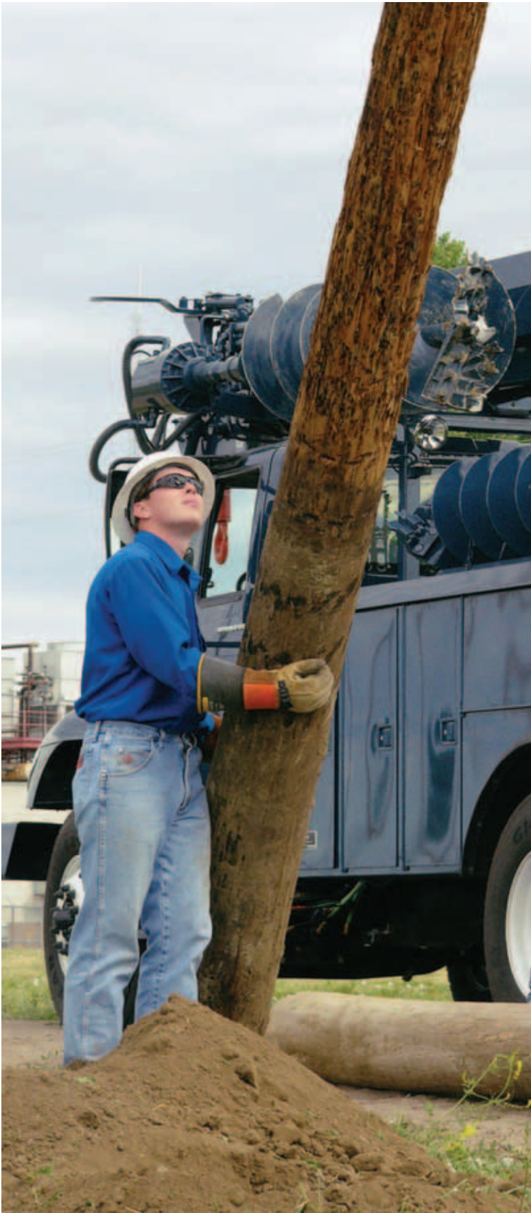
Jeff Holzer, journeyman lineworker, sets a pole in a newly dug hole. He always wears rubber gloves, safety glasses and a hard hat to protect him from accidental electrical contact.
