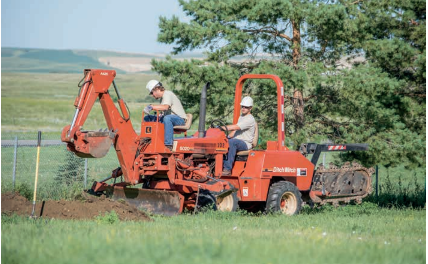
Capital Electric Linemen Matt Hagen and Braden Martin prepared an underground terminating station for hotline school at the BSC lineworker training facility in Mandan. The annual training, hosted by the North Dakota Association of Rural Electric Cooperatives, teaches linemen how to work safely around energized lines.
