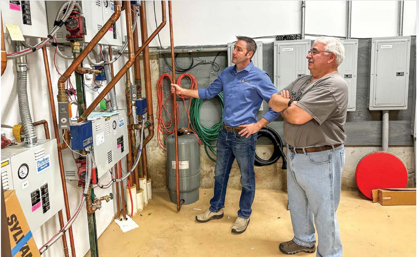
Energy Services Manager Josh Schaffner explains the cost-savings process of the heating system to Tom Thompson of the Bismarck-Mandan Rifle and Pistol Association, one of our commercial members. Our recommendations could save the association up to $500 per month by switching to our coincident peak rate and installing a controller on its boiler and ventilation fan system.
