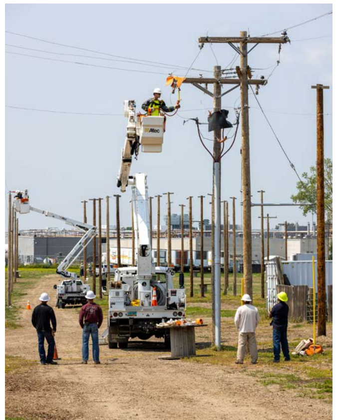
Lineworkers require intentional training to remain safe during line work in all weather conditions.
