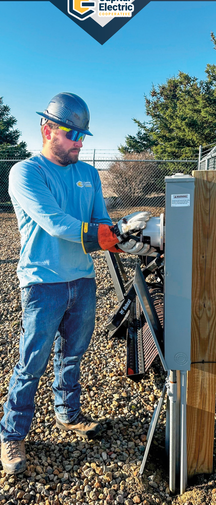
Journeyman lineworker Braden Martin replaces an existing two-way automatic communication system meter with a new digital wireless meter.
